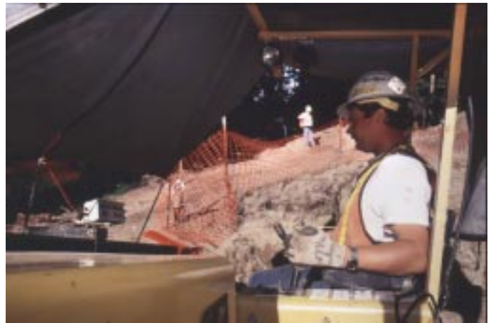
Drill operator observing the remote display information while the locator in the background tracks the tool.
