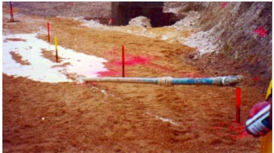
The drill head exiting from the ground at the end of the bore right on target.
