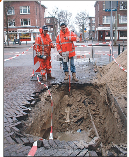
Locating is an integral part of any HDD project, but is often viewed as the “black magic” part of the operation.
